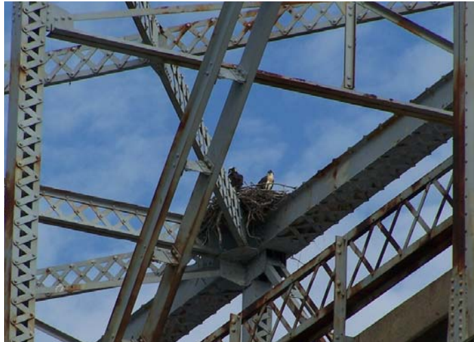
An Osprey nest on the US-68 Bridge over Kentucky Lake, taken during the 2011 Osprey survey.
